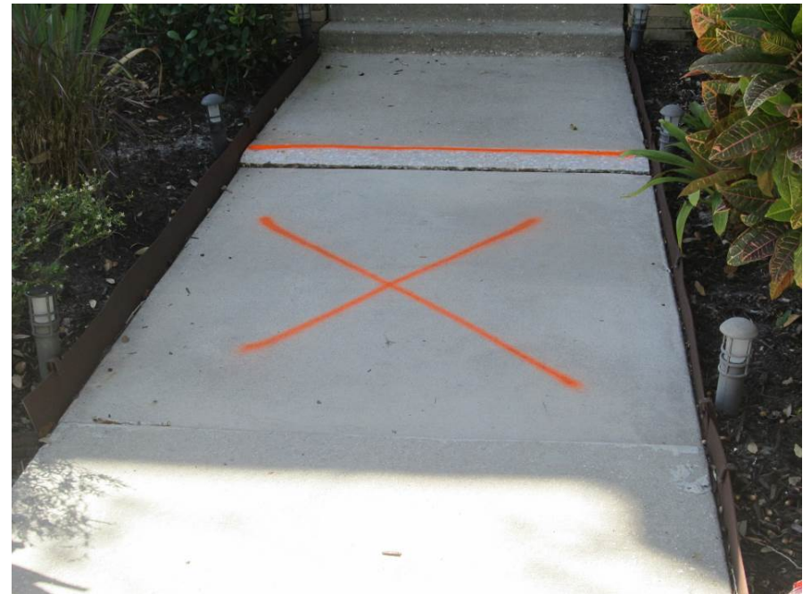
Replace 6' x 5' panel lot 104 Whitehead St
