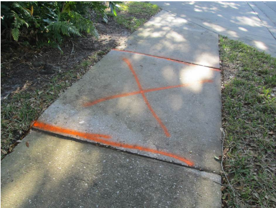
Replace 5' x 5' panel on Mallory Square adjacent to lot 60
