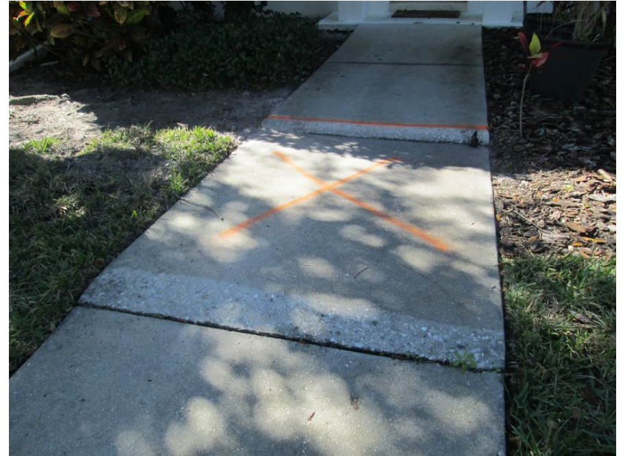
Replace 6' x 5' panel lot 129 Whitehead St
