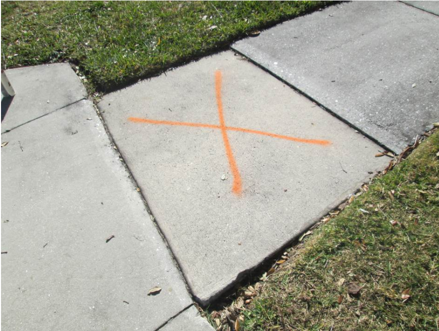
Replace 4' x 5' panel lot 130 Whitehead St
