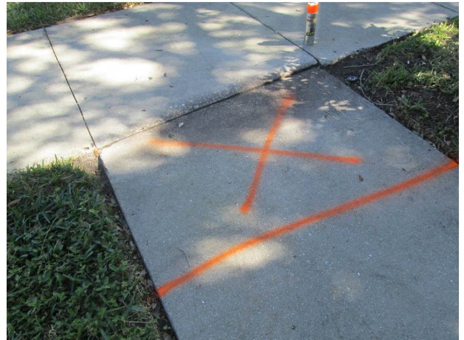
Replace 3' x 5' panel lot 129 Whitehead St
